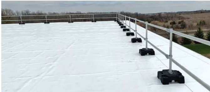
TPO roof - VSS Compact
